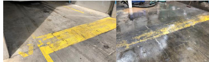
7.1- (B) & (C)- Hump at end and middle of factory
