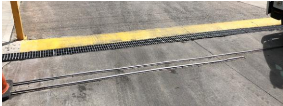
7.1- (D)- Grate Drain System-Ed of Driveway
